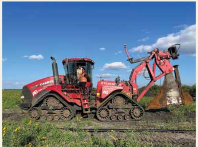
GIS Technician Sarah Chirwa works with an Agri Drainage employee to install tile at Zambia’s Nakambala Sugarcane Estate.
