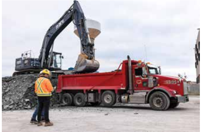
Log your loads with the simple click of a button, and easily manage your bulk material movements using SoilFLO.
