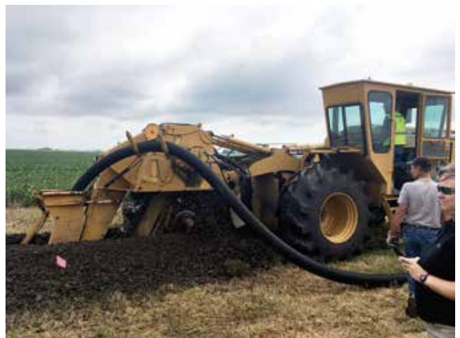
Figure 2 Iowa Batch and Build bioreactor installation by ADMC and LICA member Hands On Excavating.
