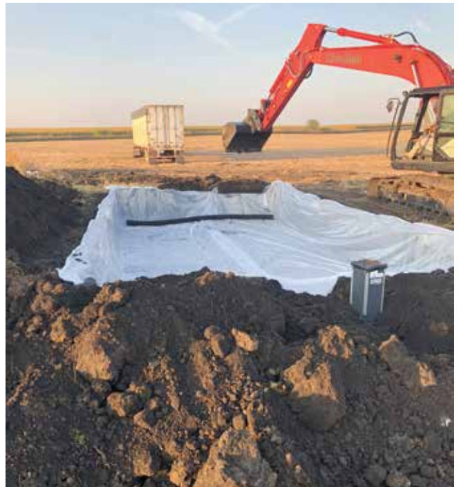
Figure 1 Installation of a saturated buffer lateral line by Illinois LICA at an ADMC partnered field day.
