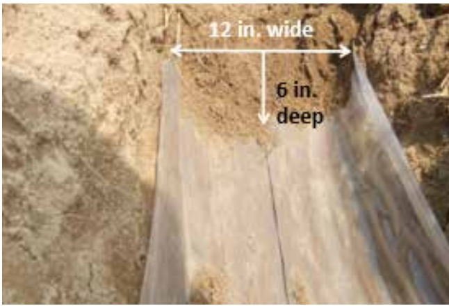
Excavated water and nutrient saving membrane, installed at 20 in. soil depths, at the base of the membrane positioned into a U-shaped trough that is 12 in. wide and 6 in. deep.
