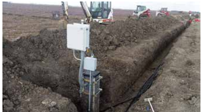
Fall 2016 field lab installation demonstrating telemetry and pump controls, as well as the underground tubing system designed to transport water samples from the control structures to the nutrient sensor. The equipment allows for a fully automated pass-through sampling system, a first-of-its-kind in the country for field agricultural research. Image courtesy of Waterborne Environmental.
