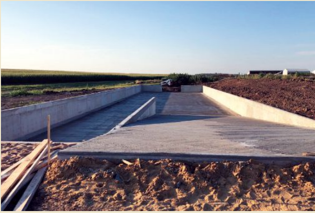
After Schell Construction excavated and leveled the area, the concrete was able to be poured for this 190-foot long, five-foot deep and 45-foot wide manure pit.
