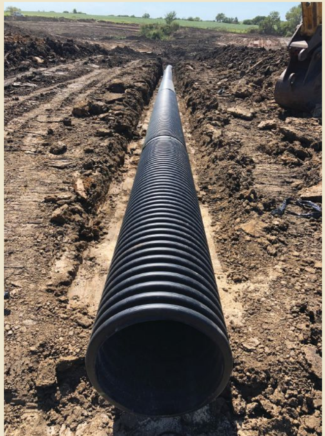
The 18-inch outlet pipe for one of two sediment ponds installed on the free-stall dairy barn project
