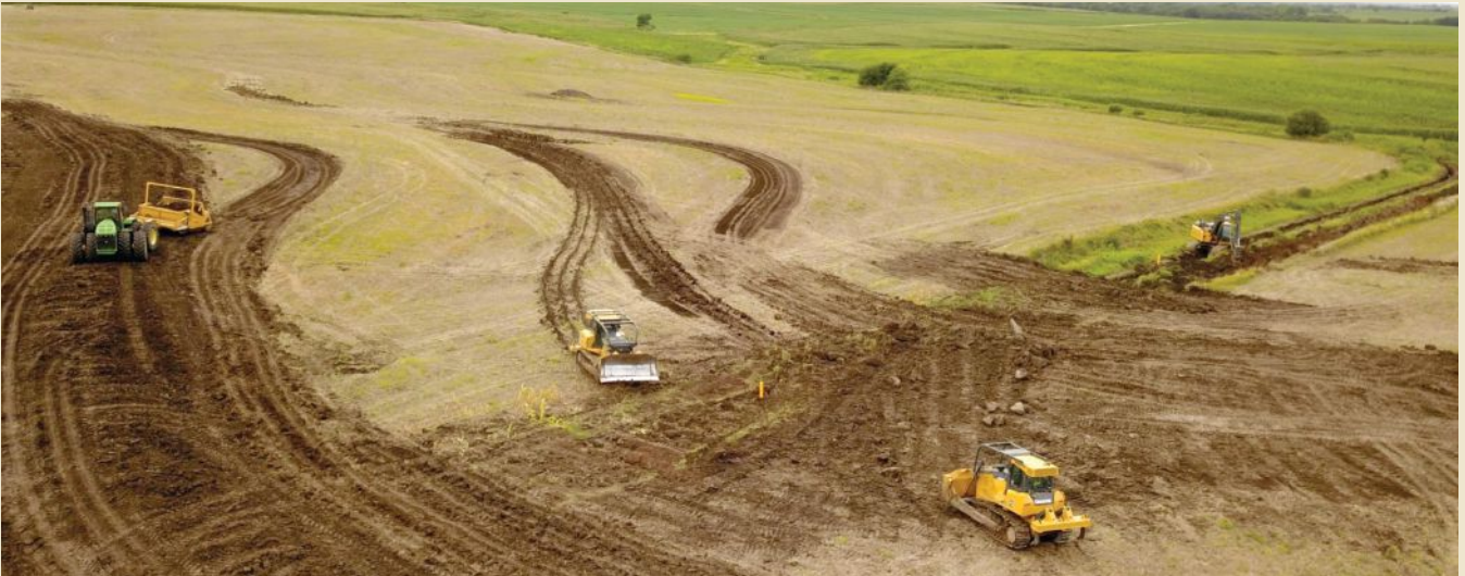
Replacing a grass waterway from the 1960's and installing underground outlet terraces
