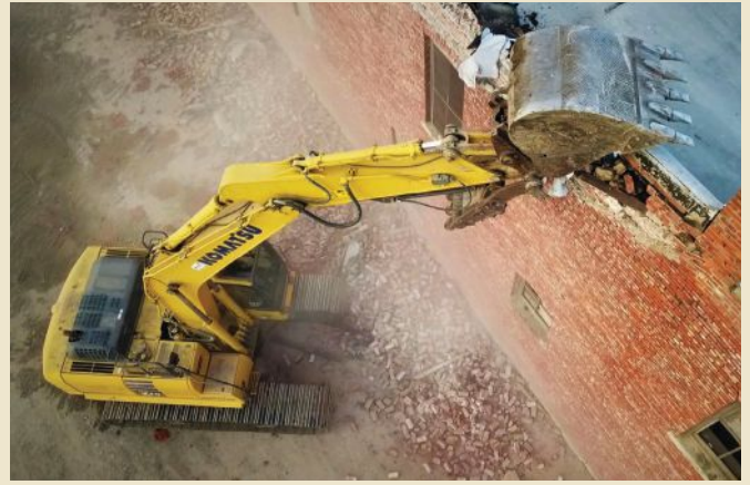
This demolition was a little tricky because Jeff had to salvage the brick for re-use in a parking lot, while separating it from the wooden roof.
