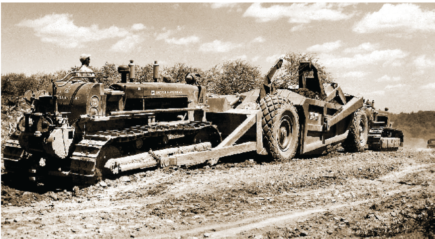
International TD24 with Bucyrus Erie cable blade pushing another TD24 and Bucyrus Erie B250 scraper. Working near Hunter, NY for I. & O. A. Slutzky, early 1950s.
