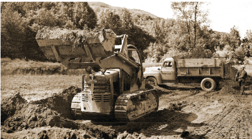
Lodover overshot type loader on International tractor working near Boiceville, NY for I. & O. A. Slutzky, early 1950s.
