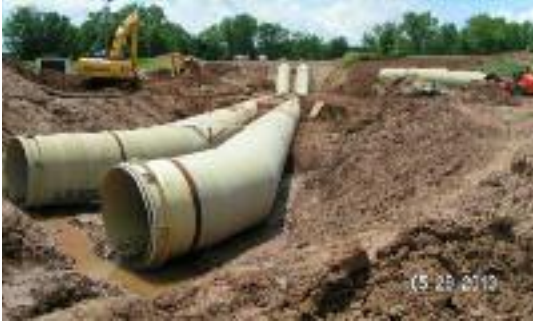
Little Bayou Meto Pump Station
